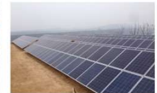
Photovoltaic project construction in Ji County for the poverty alleviation purposes
